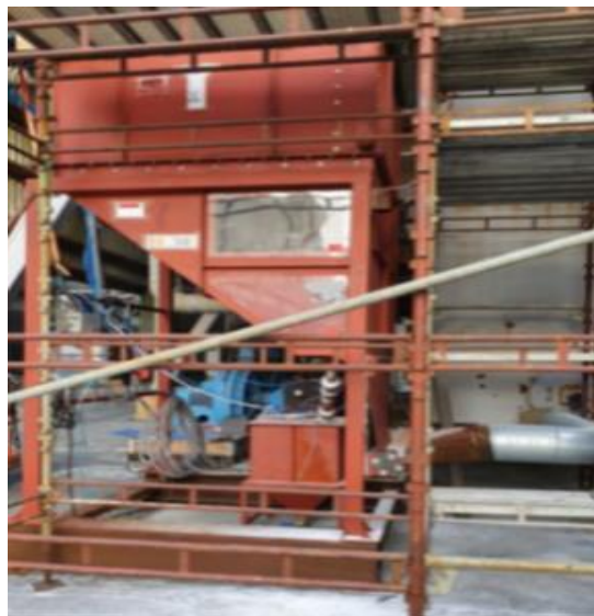
Figure 5. PIA Prototype Initial Site Test Installed at Alcoa Mosjøen.
